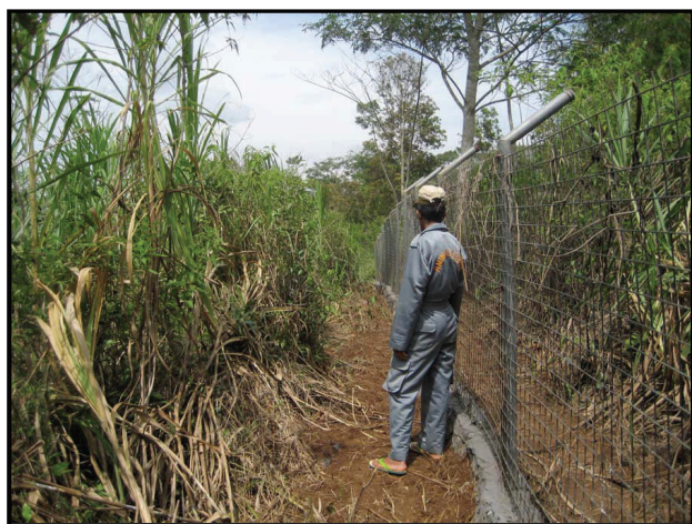
Captive breeding construction of the SV facility in Sukabumi. A subdividing fence between pen 1 and 2.
